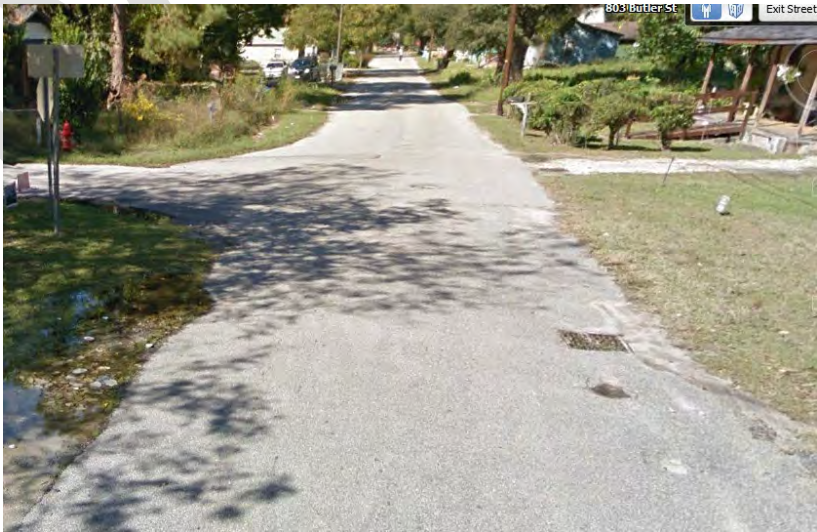
Photo 10 - Butler Street at Lincoln Street looking north. Catch basin in foreground fill with sediment. This is typical throughout the problem areas.
