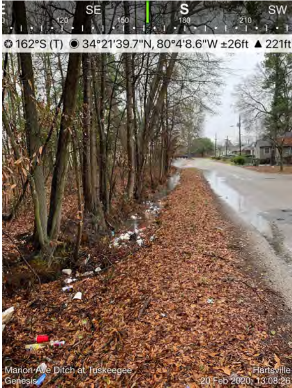
Photo 5 – Tuskegee Street – Ditch draining to outlet toward Fifth Street that is not well defined and is filled with trash/debris. This ditch enters the outlet culvert that flows toward Fifth Street. See next figure.
