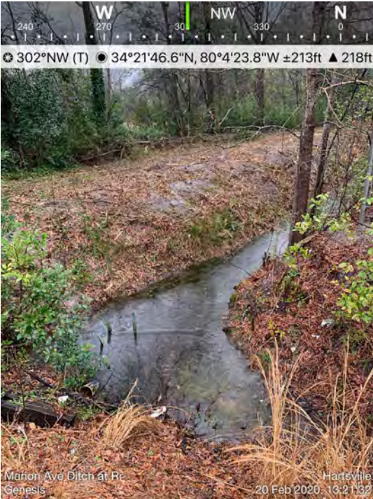
Photo 3 – Ditch just upstream of the railroad and downstream from Lincoln Avenue. This segment is also close to homes and should have channel replaced by a piped system to prevent exposure to litter and debris.
