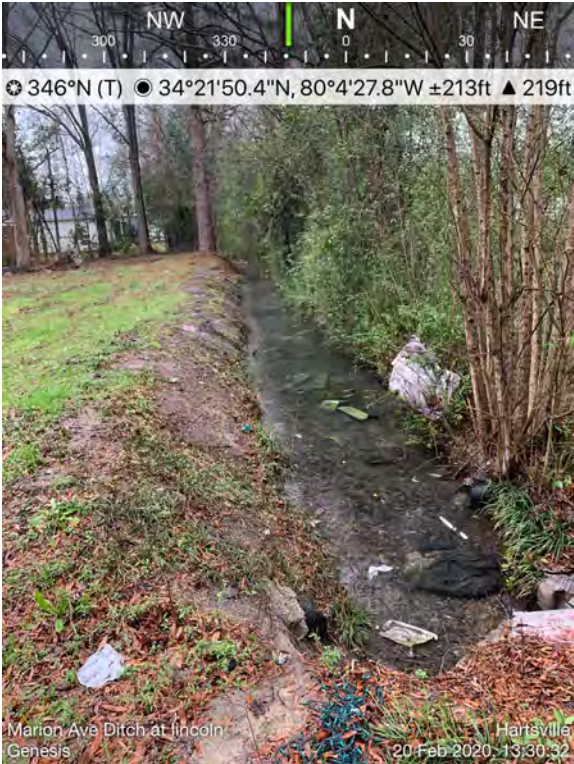
Photo 1 shows the major drainage system at Lincoln Avenue – looking upstream. Much debris can be seen within the ditches after heavy rainfall that can cause blockages within the cross culverts. The open channel needs to be replaced with a piped system to increase capacity via reduced roughness. Also, stormwater filled channels presents a health hazard allowing mosquitos and other insects a place to breed and is could be toxic.
