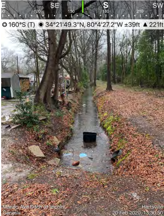
Photo 2 – Lincoln Avenue – looking downstream. Notice the proximity of the channel to the homes. This segment should have channel replaced with concrete pipe to increase capacity and reduce litter from entering the drainage system.
