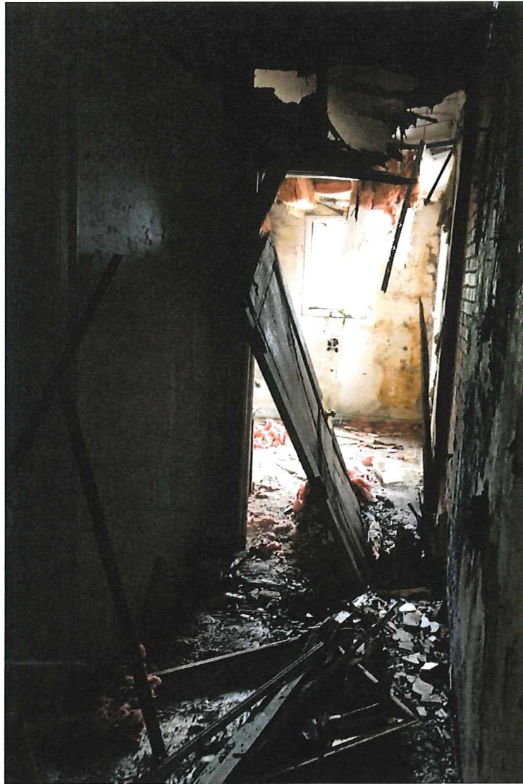
Photo 30 – Second level deterioration in corridor
