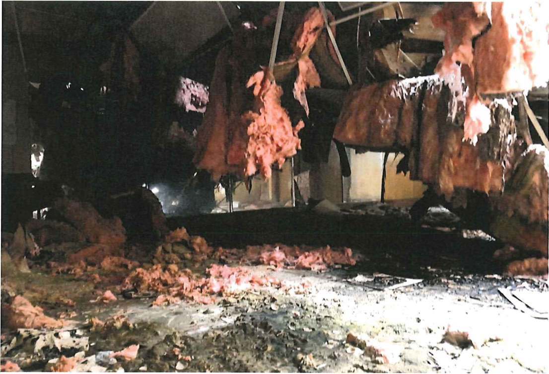
Photo 33 – Second level deterioration
