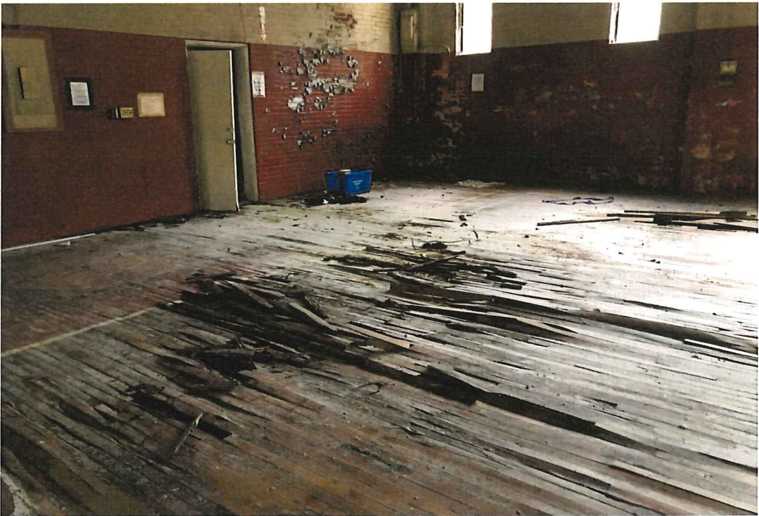
Photo 36 – Deteriorated c.1981 floor, drill hall
