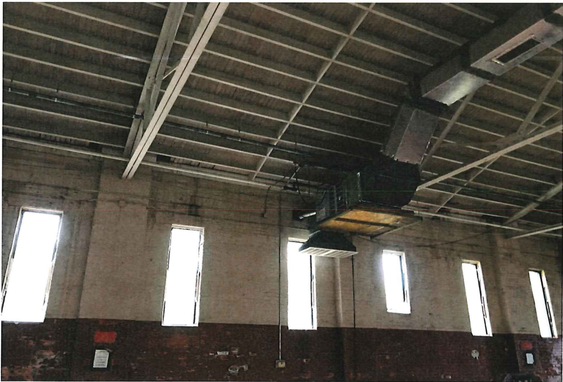
Photo 38 – HVAC unit penetrating wall, drill hall looking east
