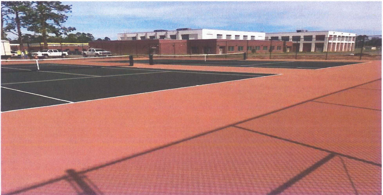
College of Coastal Georgia – Brunswick, GA – 2011 - Gary Strickland, Supervisor, 912-279-5835 – We removed the existing tennis courts and reconstructed 12 new courts along with 12 drinking fountains, sidewalks, and lights.
