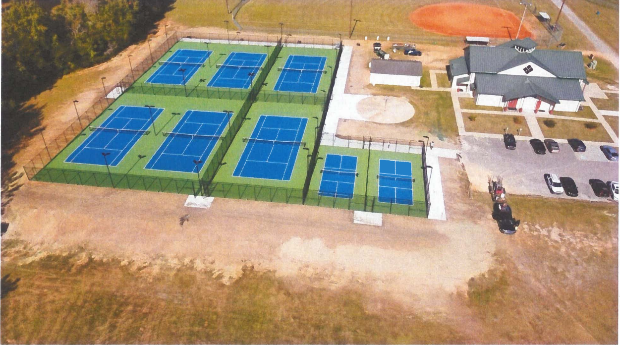
Cook High School – Adel, GA – 2019 – JCI Contractors - Adam Hurst - Our scope of work involved the construction of eight tennis courts and included fine grading of the subgrade, placing, compacting and fine grading the GAB, placing and compacting the tennis court asphalt, curb around the perimeter of the tennis courts, tennis court fencing, sidewalk between the tennis courts, tennis court windcreens, tennis court equipment, and surfacing & striping of the tennis courts.
